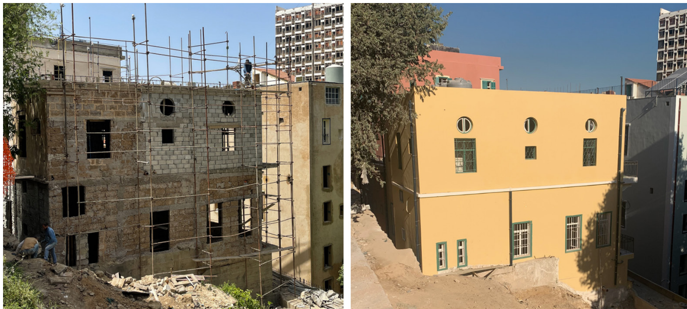
A sandstone facade of heritage value, before and after undergoing its rehabilitation under the Rmeil Cluster project (n.d.)
