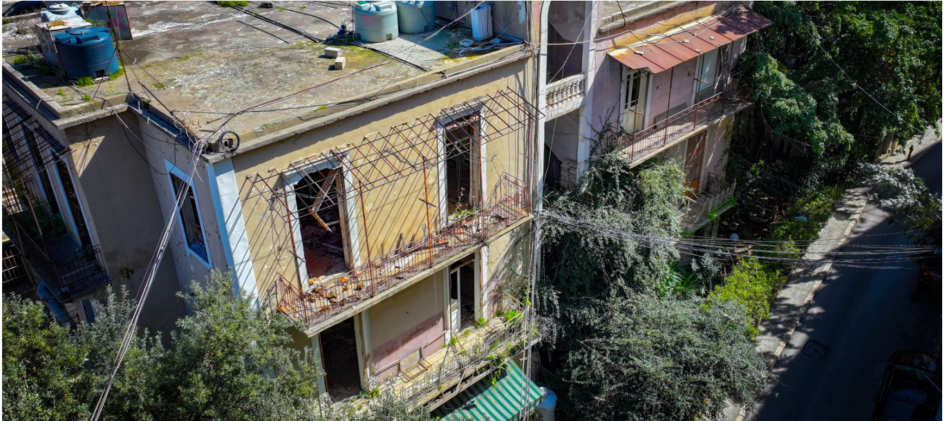
A building of heritage value from the 1930s in Rmeil before its rehabilitation under the BERYT project (UN-Habitat Lebanon, 2022)
