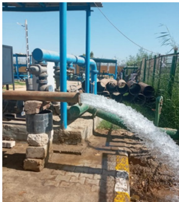
Fresh water from the River Bank Filtration (RBF) system.
